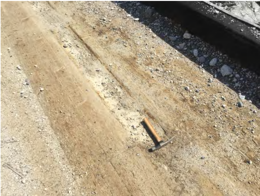
Heavily Worn Running Plank
