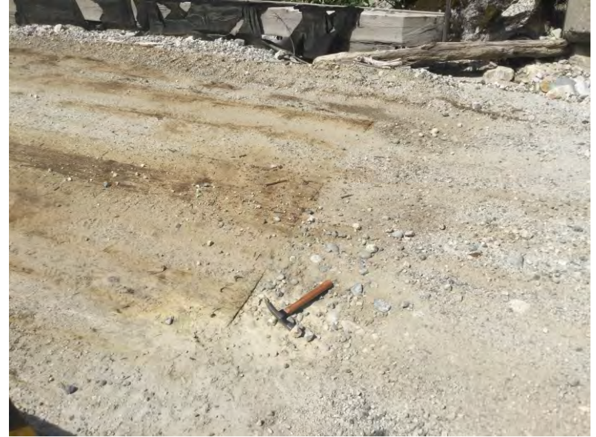
Left Approach Pothole Adjacent to Deck
