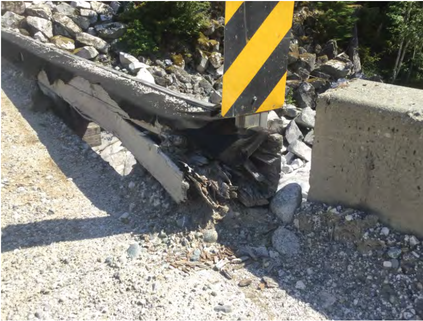
Right Abutment Damaged Guardrail
