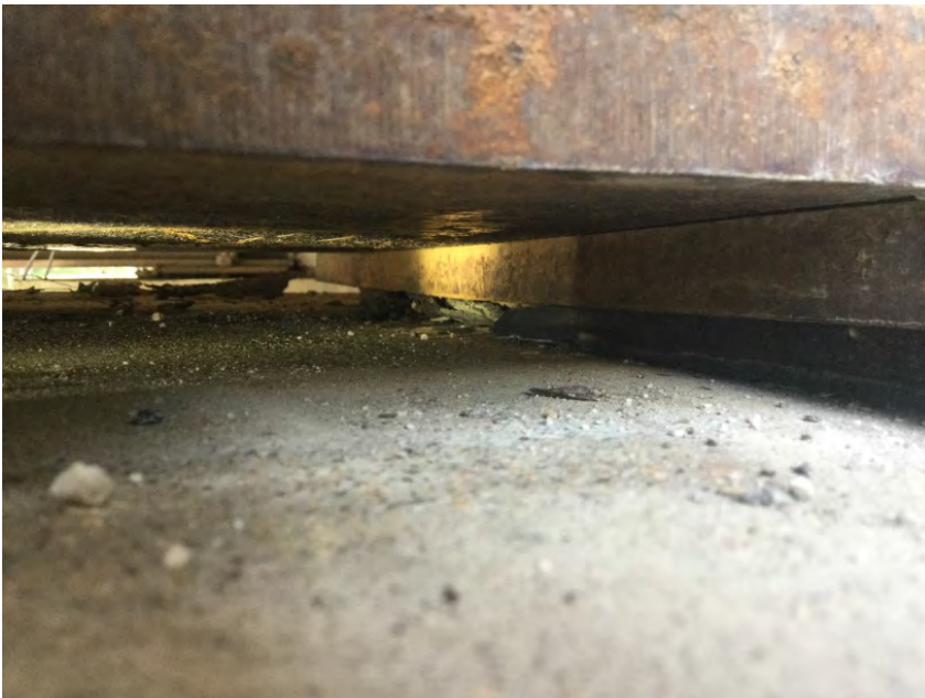
Damage to Right Abutment Upstream Bearing
